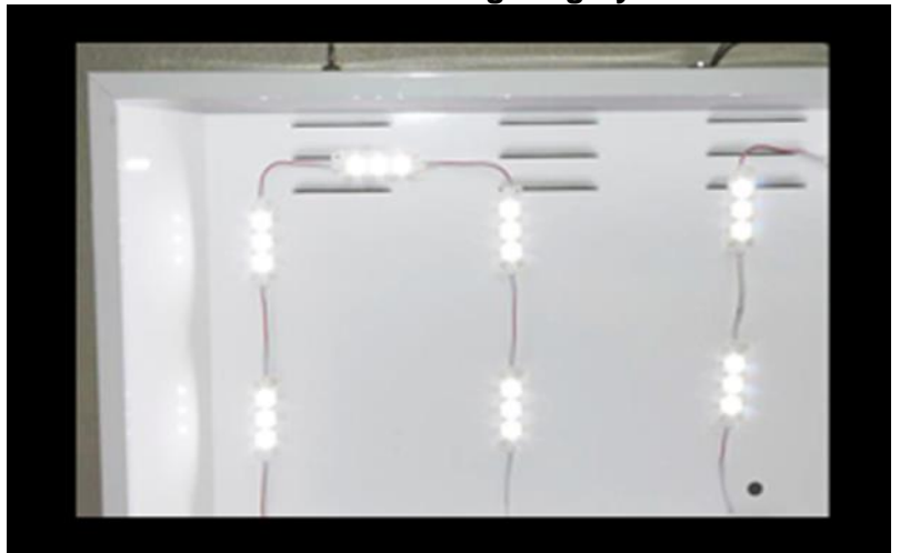
Inside LED Lighting System
